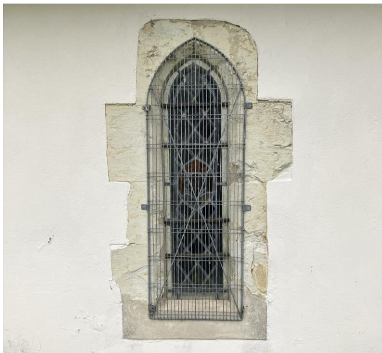
above: South aisle, window west of porch. Note very poor condition of masonry window dressings.
