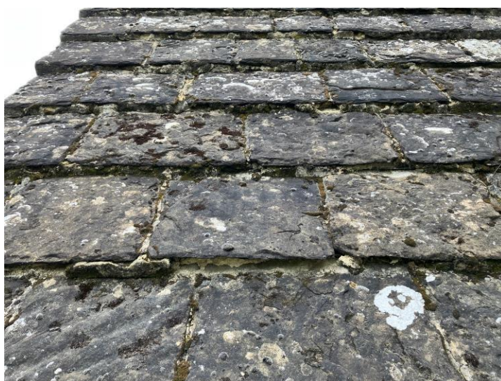
above: Defective pointing between Horsham stone slates on south aisle roof.
