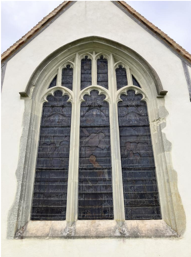
above: The Chancel east window. Note uniform-looking masonry, which is, in fact, cement-based repair material.
