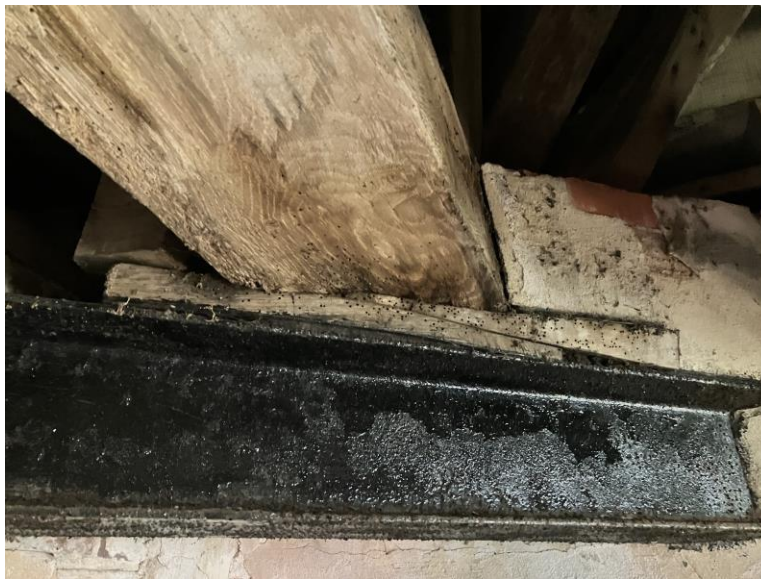
above: Evidence of beetle activity, south-western corner.
