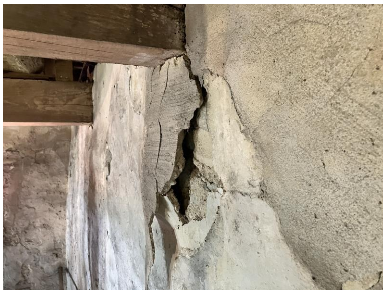
above: Loose plaster in belfry
